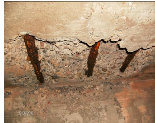
Figure 41 Corrosion of steel in RCC
